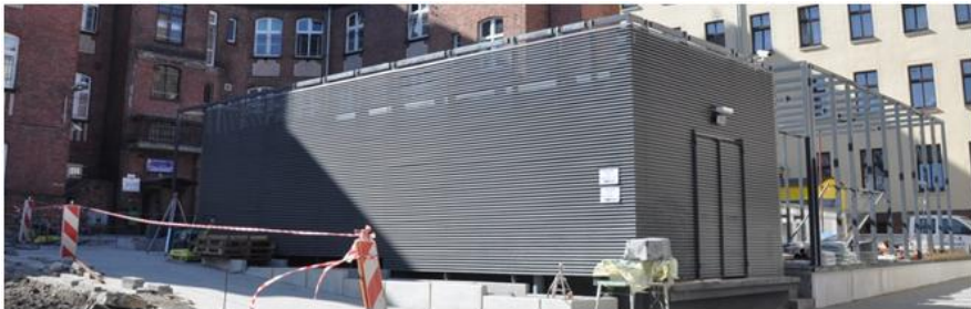
Fig. 4. Extension and renovation project of the St. Joseph Hospital in Poznan. Admission room and oxygen room projects and an actual view of the oxygen room, currently under development.
